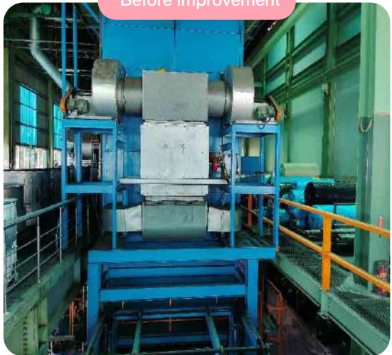
Caption : Before improvement: There was no protective barrier in the filter disassembly operation area of the padding machine.
