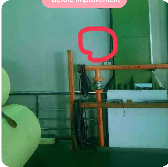
Caption : Before improvement: There was no natural gas detector above the natural gas switch.
